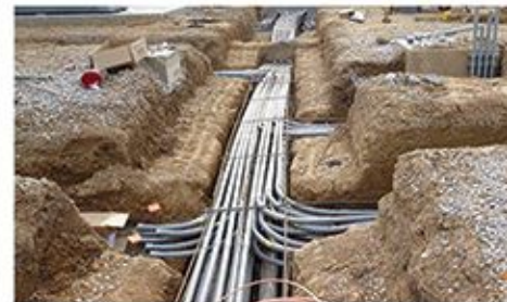
Under Ground Wiring
